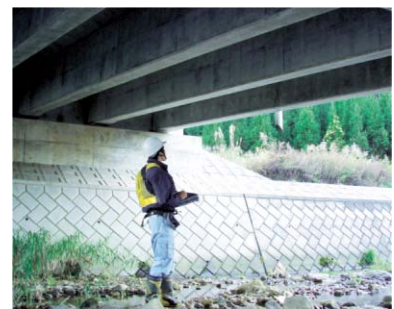
Workers use mobile computers to efficiently input the results of bridge inspections.
