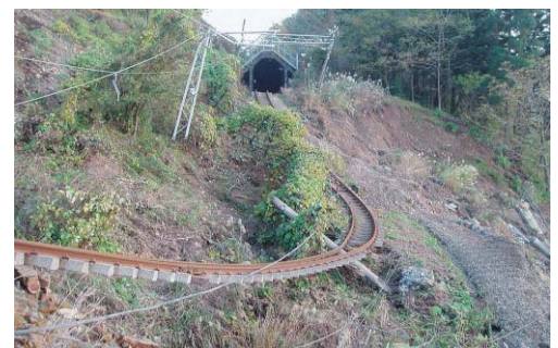
The collapsed western end of the Tenno Tunnel
