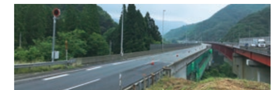
Kan-Etsu Expressway Anogawa Bridge, where deck slab renewal work will be carried out using the SDR system
