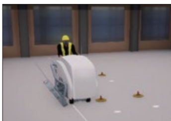
(1) In advance, floors are dismantled into slabs using diagonal cutters inside the enclosed building.
