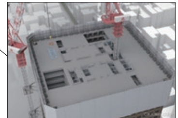
(4) The lowerable scaffold, which serves as the demolition work area, is lowered to the next floor, and steps (1) through (3) are repeated.
