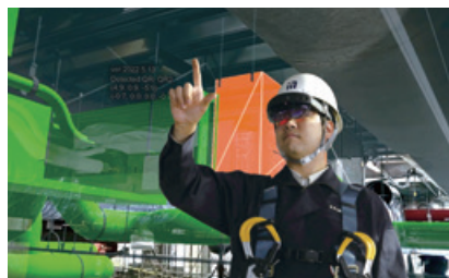
Checking the construction alignment by overlaying the actual product and BIM (BIM utilization)
