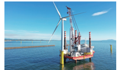
Construction of Offshore Wind Farms at Akita Port and Noshiro Port ▶ Page 41
