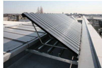
PV solar air panels
