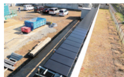
Solar panels used at construction sites
