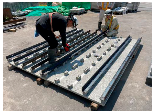
Photo 1 仮組みヤードでの大判化の様子 (Assembling of CUCO-SUICOM Formwork at Site)
