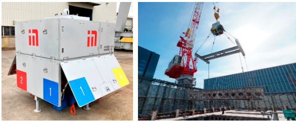
Fig.25 4点自動吊上げ装置とスラブ揚重状況 (4-Point Automatic Lifting Device and Slab Lifting Situation)
