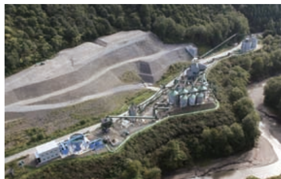
Blue hydraulic shovels, etc., are used (upper right) Taking into account the colors of plants at construction sites (below)
