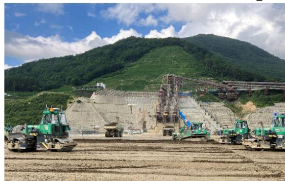
Naruse Dam Construction Project progressing with the use of automated construction technology A 4 CSEL (Akita Prefecture)
