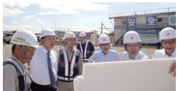
Tour of a construction site in Taiwan by an outside director (third from right: Koji Furukawa)
