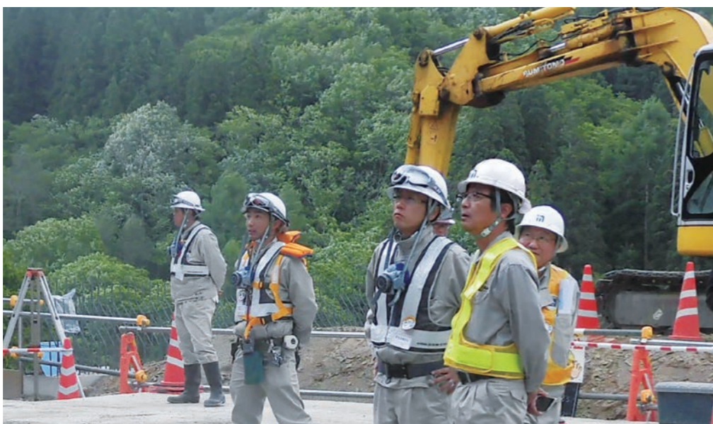
Hiroshi Shoji (foreground), General Manager of Tohoku Branch, observes construction at the Reconstruction Support Roads project.
