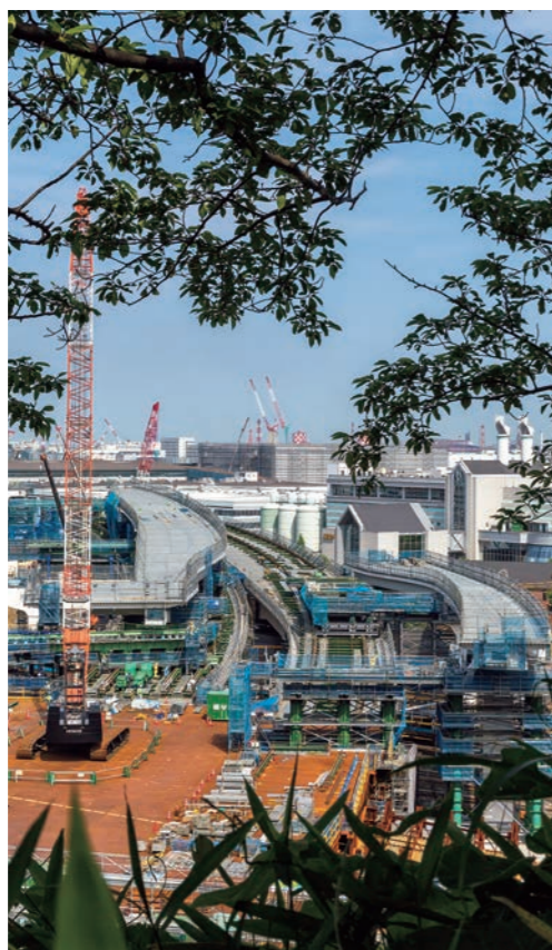
New junction for the Yokohama Circular Northern Route, Metropolitan Expressway (Koyasudai, Kanagawa-ku, Yokohama–Kishitani, Tsurumi-ku, Yokohama)
