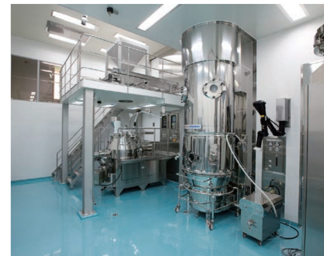
Facilities at the second solid dosage building of the Kagamiishi Plant of Nipro Pharma Corporation.
