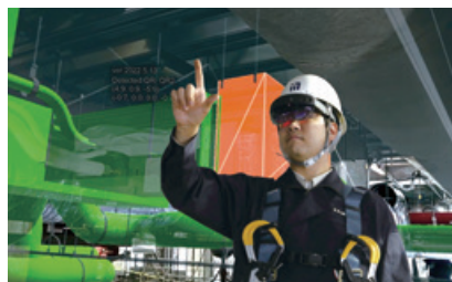
Checking the construction alignment by overlaying the actual product and BIM (BIM utilization)
