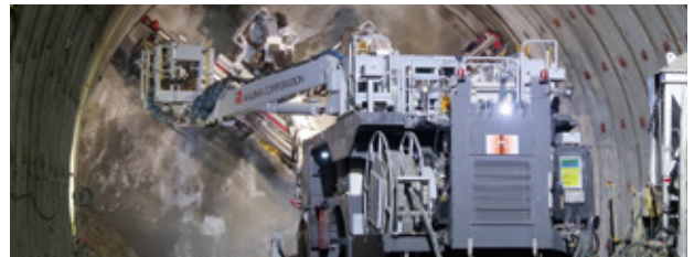
A 4 CSEL for Tunnel
