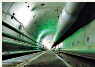
Gas pipeline inside the tunnel
