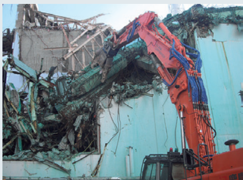
Tearing down a damaged building at the Fukushima Daiichi Nuclear Power Plant. (Photo: Tokyo Electric Power Company)
