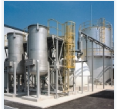
The world's first bio-gas fuel cell power plant equipped with "METAKLES".
