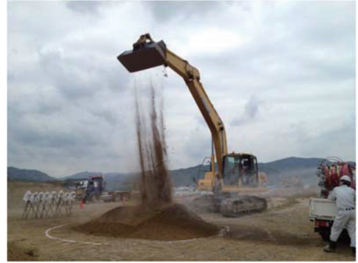
Photo 4 バックホウ作業時の噴霧状況 (Spray Situation at the Time of Backhoe Work)
