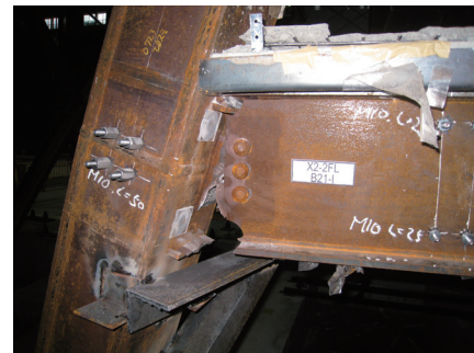
梁の破断状況 Fracture of Beam End Connection
