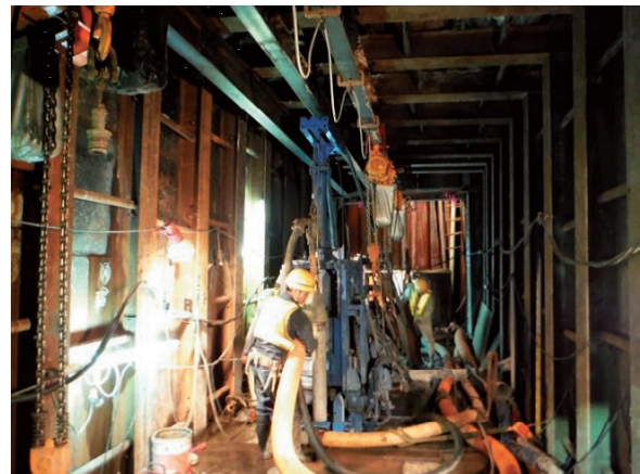
狭隘な導坑内でのBCH工法の施工状況 Construction Situation of BCH Method in a Narrow Guide Hole
