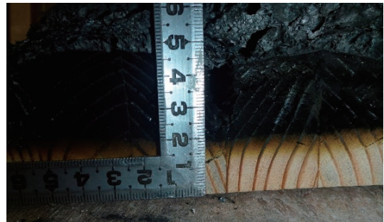
Photo 6 加熱試験後の残存厚さ, No.2 (Residual Thickness After Heating Test, No.2)
